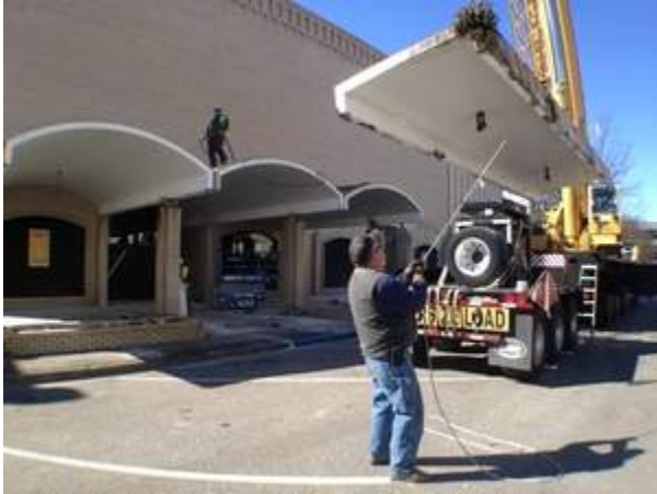
Workers remove sections of the canopies at the old Belk Building on Dexter Avenue on Friday morning.
